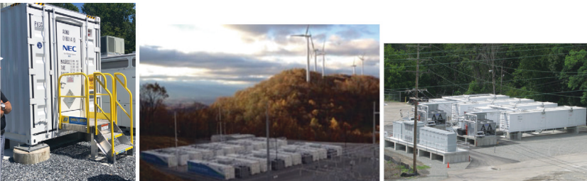
Figure 15. (left) A load shifting battery facility at a sub-station south of Saratoga Springs, New York, 2019; (middle) a 16 MWh battery facility in West Virginia, USA to smooth wind power and to shift the load, and (right) a former battery facility in Binghamton, NY.
